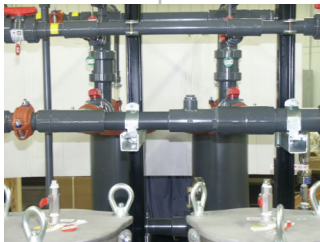
PVC Paint Manifold
